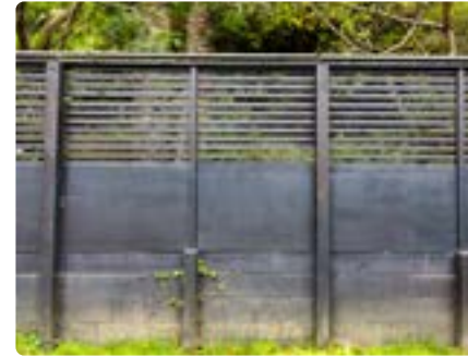
An existing fence, increased in height to more than 1.8 metres with a rolling attachment.
