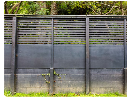
An existing fence, increased in height to more than 1.8 metres with a rolling attachment.
